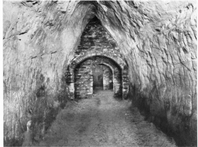
Tunnel Road East mine: this north-south inverted V profile tunnel ceiling, along with built-brick support, suggest a joint or line of weakness in the rock. Clearly the miners has experienced 'overbreak' in this area, more sand having fallen from the ceiling than was intended.
